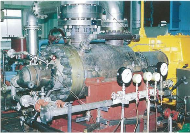
Barrel casing boiler feed pump 2,925psi-2,980 U.S.gpm-5,610min -1 -7,240HP Petacalco Power Plant(Mexico), 350MW×4units
