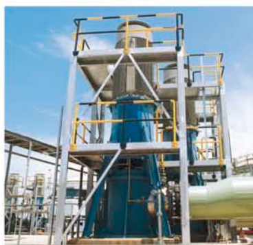
Sea water cooling pumps, Singapore (Size:800mm, Driver:790kW)
